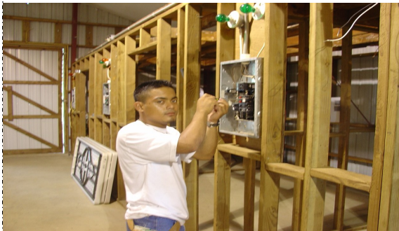
Student performing practical tasks in the electrical workshop.
