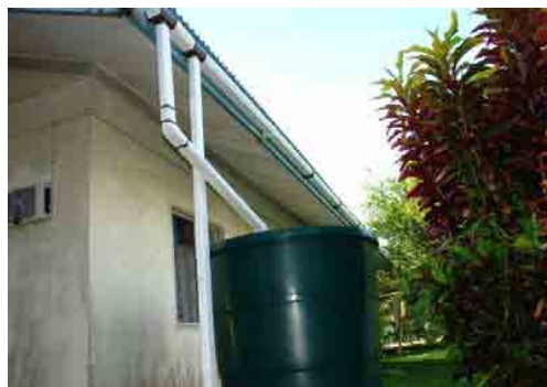
A sample of a rain catchment system
