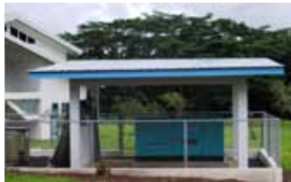
The newly installed generator at the national campus with its newly constructed housing.
